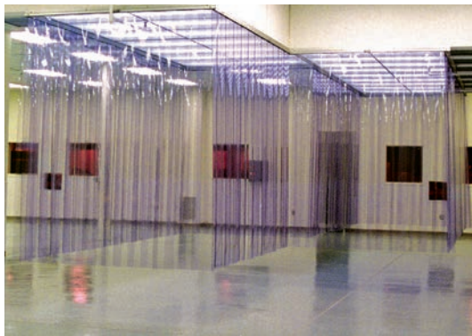
This enclosure is in As Built state, before equipment and materials are moved in. Notice that it is within an existing room and takes advantage of the air conditioning infrastructure that is already installed. Cleanrooms are certified by the manufacturer in an As Built state.
