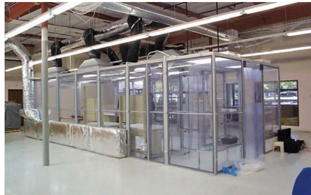
Rather than ceiling plenums and air chases in the walls, this room uses an elaborate system of ducting to recirculate air leaving the room, and bringing it back in through the ceiling to pass through the HEPA filters before re-entering the room. The gowning area on the right end of the room provides technicians a place to gown before entering the main cleanroom, reducing the risk of contamination.
