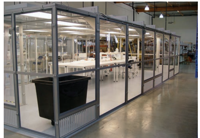
A well-organized cleanroom includes attention to process flow. Make sure furniture and equipment do not hinder air flow. Materials should come in one end and go out the other.
