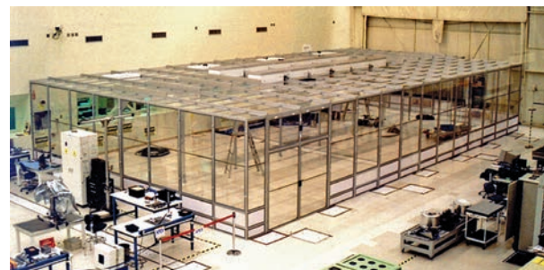
Modular cleanrooms as large as 5,000 square feet, and even larger, are often required for assembly lines, packaging operations and other environments.
